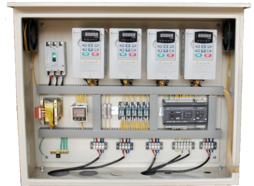
Multiple inverter systems inside layout
