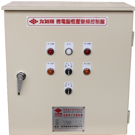
Standard inverter control panel (Duplex operation)
